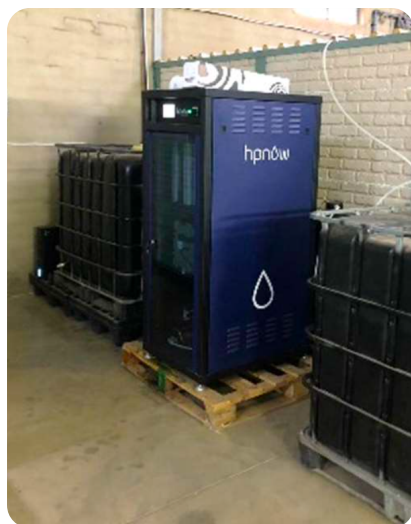
Figure 1: GOgen™ system installed at a greenhouse facility.
